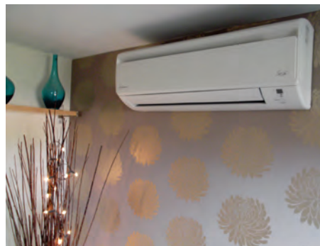
AIR-CONDITIONERS IN BEDROOMS AND LIVING ROOM
